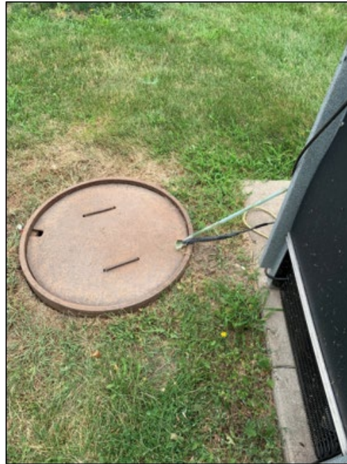
Autosampler hose enters manhole
